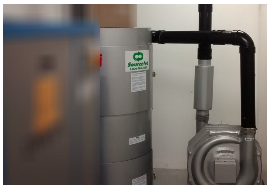
Sourcetec Detail Vacuum System
